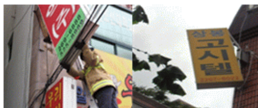
Fig. 1 Failure of sign structure
