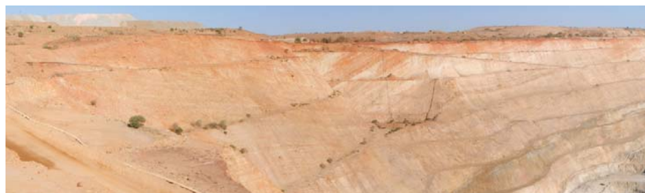
Fig. 2 Photograph showing condition of slopes in highly weathered siltstone – effectively zero slope failures 20 years after excavation
