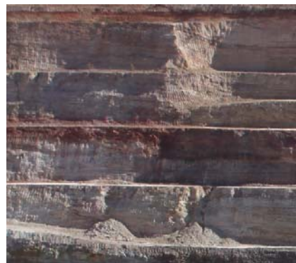
Fig. 3 Photograph showing two ‘rare’ localized 10 m high wedge failures in lowest bench of weathered siltstone
