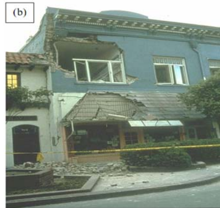
Fig. 3 (b) Front elevation damage dates in 1989 Loma Prieta earthquake
