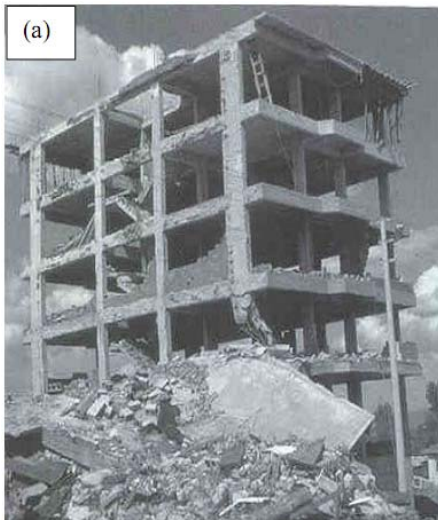
Fig. 3 (a) Column failure dates in 1999 Kocaeli earthquake
