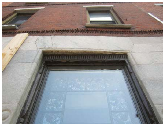
Fig. 3 Bulge at window opening
