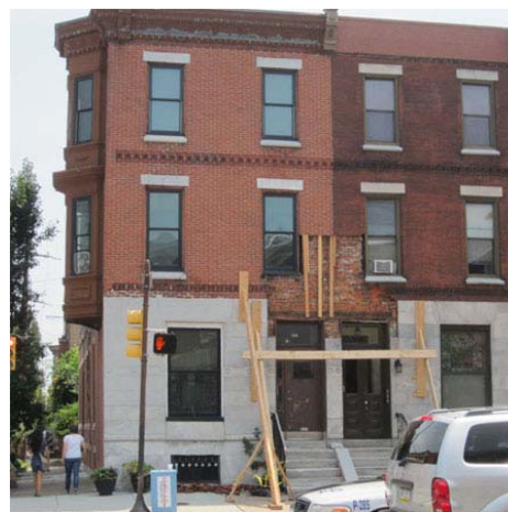
Fig. 1 Brick wall damage
