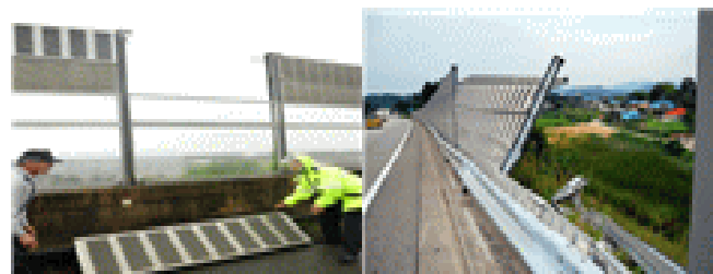
Fig. 1 Failure of soundproof wall
