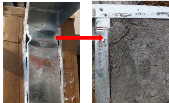
(c) Local buckling of W-3 CFS
