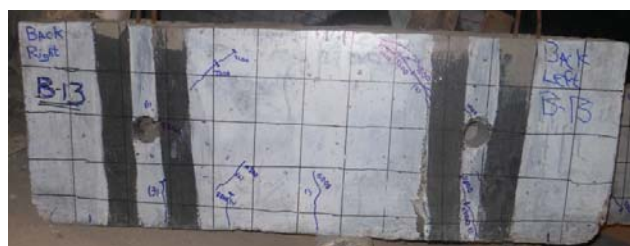
Fig. 12 Crack pattern of beams with opening at NA
