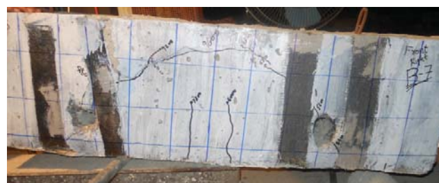
Fig. 11 Crack pattern of beams with opening below NA
