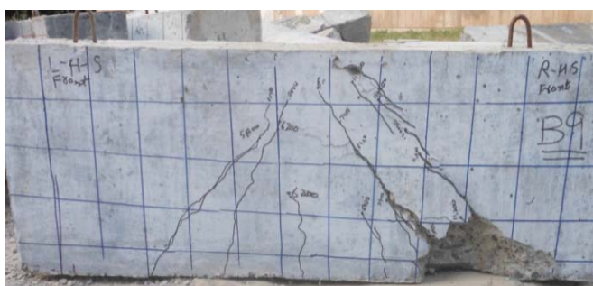
Fig. 9 457mm (18in) deep beam crack pattern
