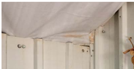
Fig. 14 Sharp edges in cladding [15]
