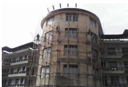
Fig. 2 Reconstruction due to original unreasonable design
