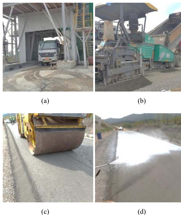
Fig. 2 Construction process of RCCP (a) Mixing and transportation, (b) Paving, (c) Compaction, (d) Curing
