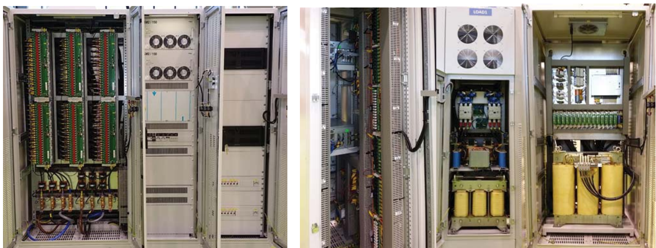
Fig. 4 LOAD laboratory unit cabinets
