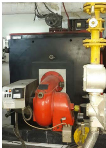
Fig. 5 Heating system serving to four buildings in Antpark campus
