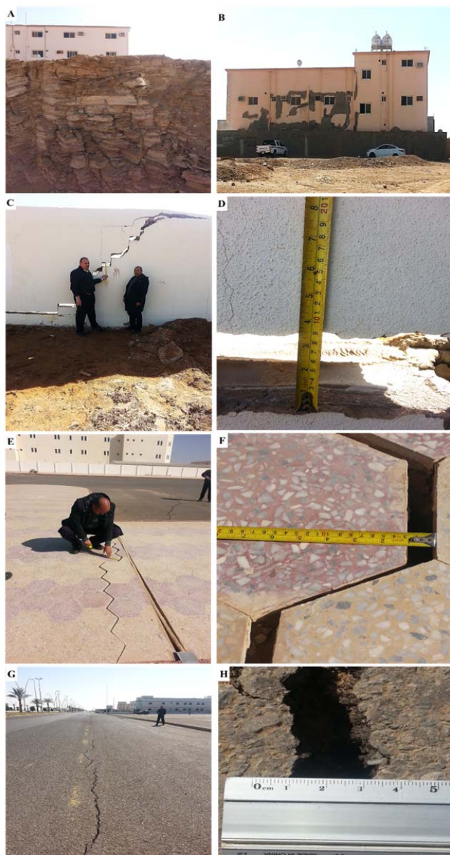
Fig. 2 Some effects of expansive shale: (A & B) longitudinal cracking and failure in housing, (C & D) boundary wall, (E & F) walkways and (G & F) roadway, Tabuk, KSA
