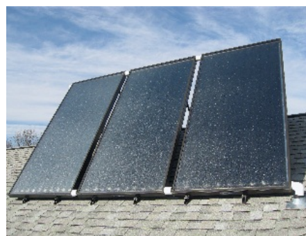
Fig. 1 Flat Plate Collector
