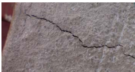
Fig. 8 Example of plastic shrinkage cracking
