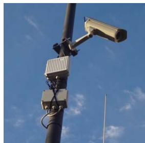
Fig. 7 An installed smart camera and the ETSI MSM Gateway installed on an existing pole during Montecatini trial
