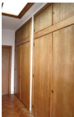
Fig. 9 Built-in furniture in limba at House Janssens (1934, Antwerp) by Léon Stynen, O. Pauwels & M. Jaenen [22]
