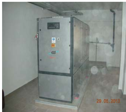
Fig. 5 Cogeneration unit 55kW
