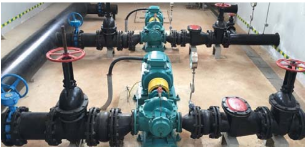
Fig. 1 Circulating Water Pump
