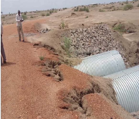
Fig. 6 Severe cracks and potholes on embankment edges due to water erosion
