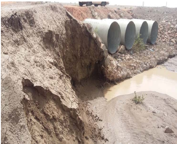
Fig. 7 Collapse and failure of wing walls embankment due to water scouring
