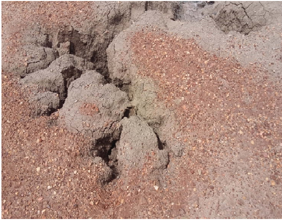
Fig. 10 Sever cracks and potholes on Subbase and embankment layers
