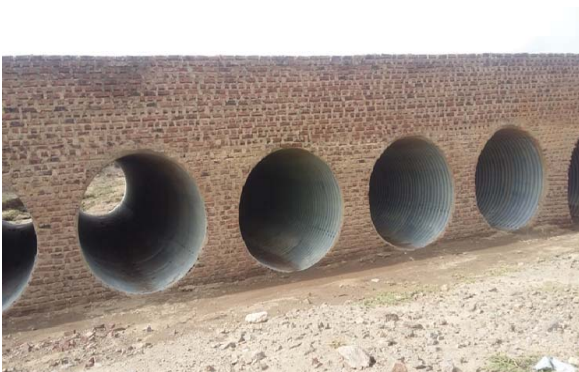
Fig. 11 Head and wing walls of the Fresh crossing are in good condition
