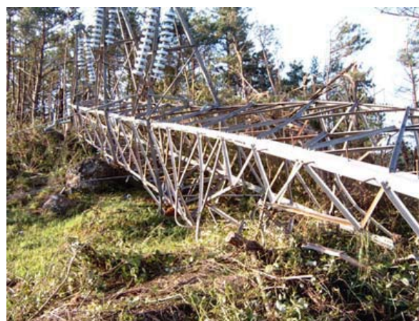
Fig. 1 The collapse of transmission tower by the typhoon ‘MAEMI’
