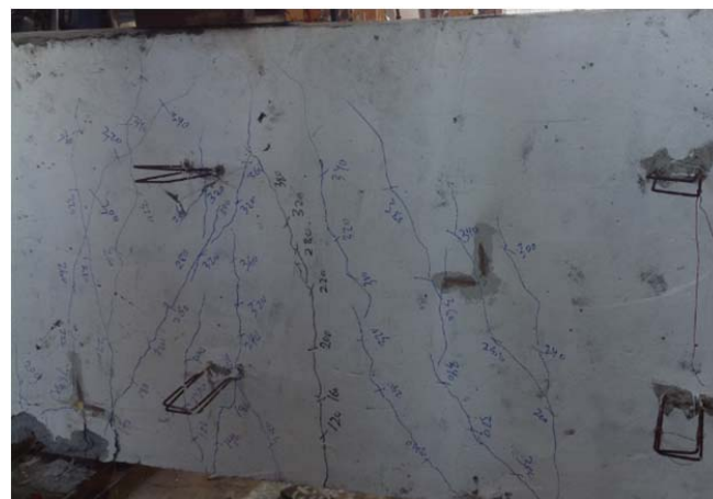
(a) Typical shear crack patterns for panel GS5 along the height of the concrete wythe
