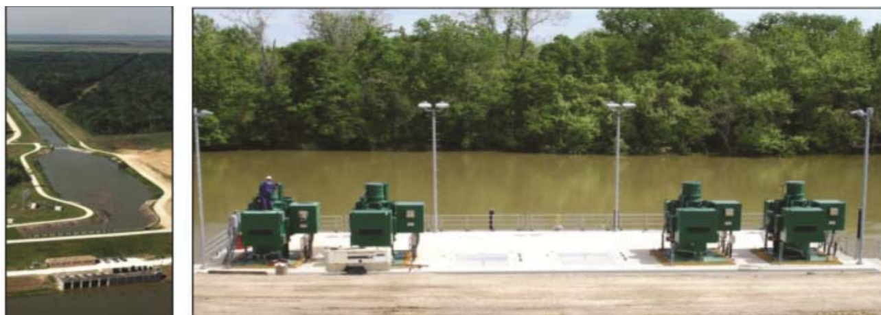
Fig. 6 Site location's existing Pump station
