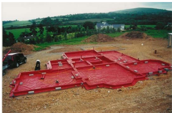
Fig. 5 Continuous radon barrier placed within the insulation layer covering the ground surface of a building. The membrane is extended to the outer side of the exterior wall and covers foundations, including foundations supporting interior walls
