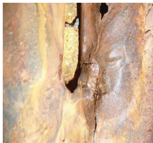
Fig. 1 Cracks at fin tip of tubes membrane
