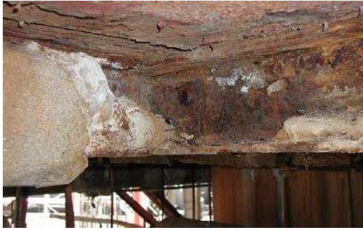
Fig. 4 Crack development in concrete structure due to fire
