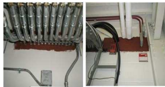
Fig. 9 Fire penetration protection system
