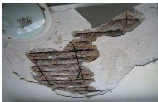
Fig. 3 Spalling of concrete
