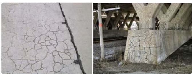
Fig. 4 ASR damage in highway projects [4]
