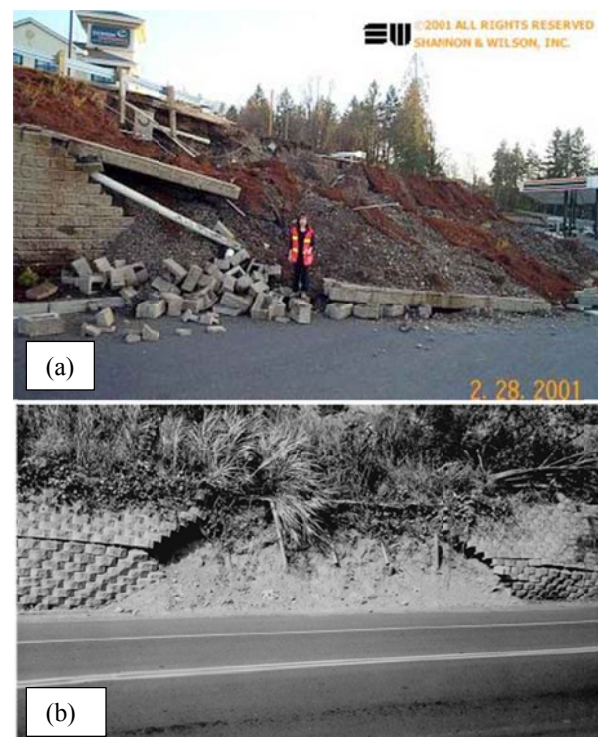
Fig. 1 Collapsed Reinforced Earth Walls During Earthquakes. (a) Extended Stay Hotel MSE Wall-Seattle collapsed after the Nisqually earthquake (USA-PEER 2001), (b) Collapsed Wall at Highway 129 after Chi Chi Earthquake [5]
