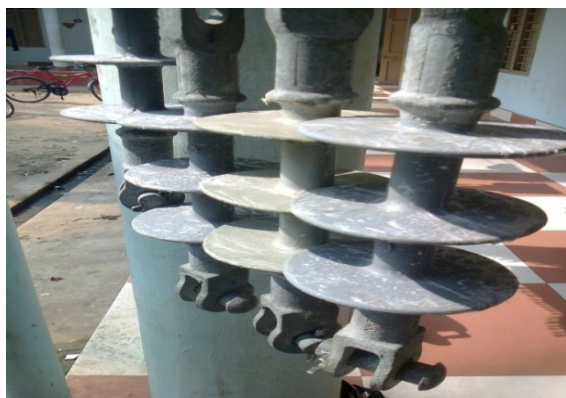
Fig. 5 11kV Specimen under urea pollution
