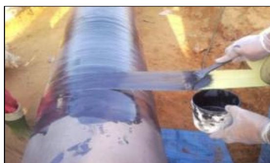
Fig. 6 Wrapping process of Kevlar tape repair system
