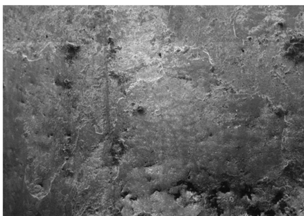
Fig. 5 Surface of steel embedded in concrete GBFS subjected to chloride ions
