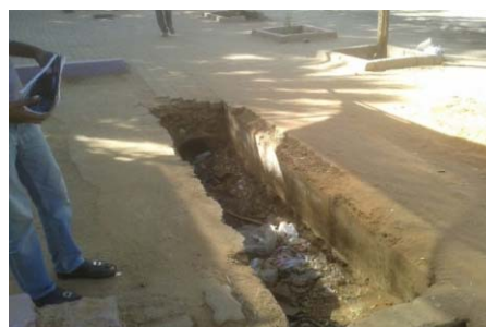
Fig. 5 Side drain of damaged cover full with debris in Alarbeen road
