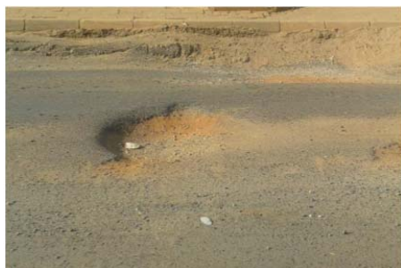
Fig. 2 Severe rutting leading to large potholes in Algaba road
