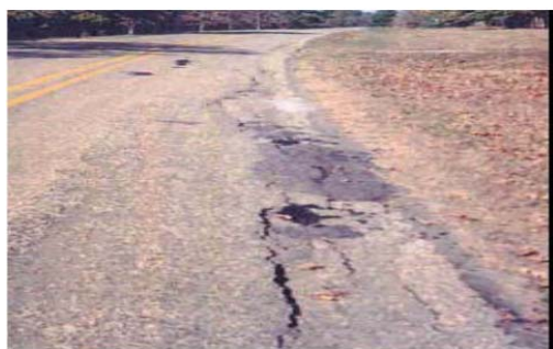
Fig. 1 Longitudinal cracking and failure, [19]
