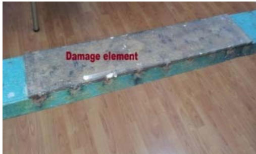
Fig. 4 Damage element in beam
