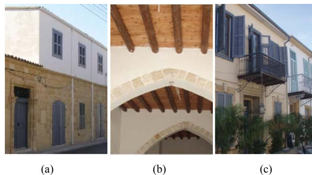
Fig. 10 (a) Load bearing stone and mud-brick walls, (b) Traditional flat roof, (c) External shutters in windows of traditional buildings
