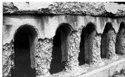
Fig. 1 Typical example of concrete deteriorated from freeze-thaw actions. (Non-air-entrained concrete railing, PCA vol. 19/1 1998)
