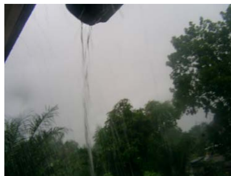
Fig. 3 Water falling from the roof gutter
