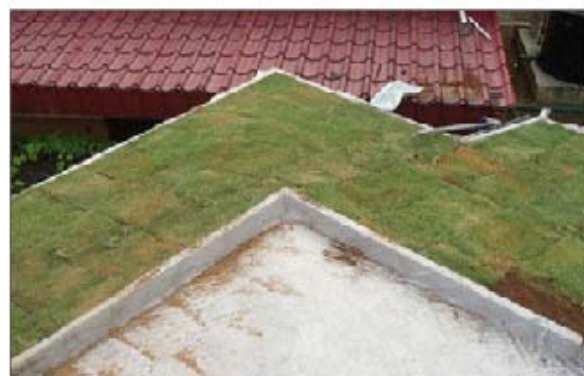
Fig. 1 Layer of geotextile materials (white sheets) placed underneath the soil layer and vegetation in a green roof system
