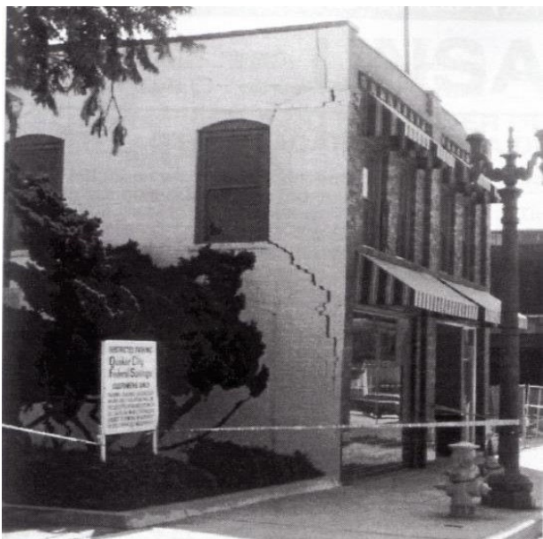
Fig. 6 Example of a crack pattern in the side wall of a masonry building documented in the ATC-20 series [29]
