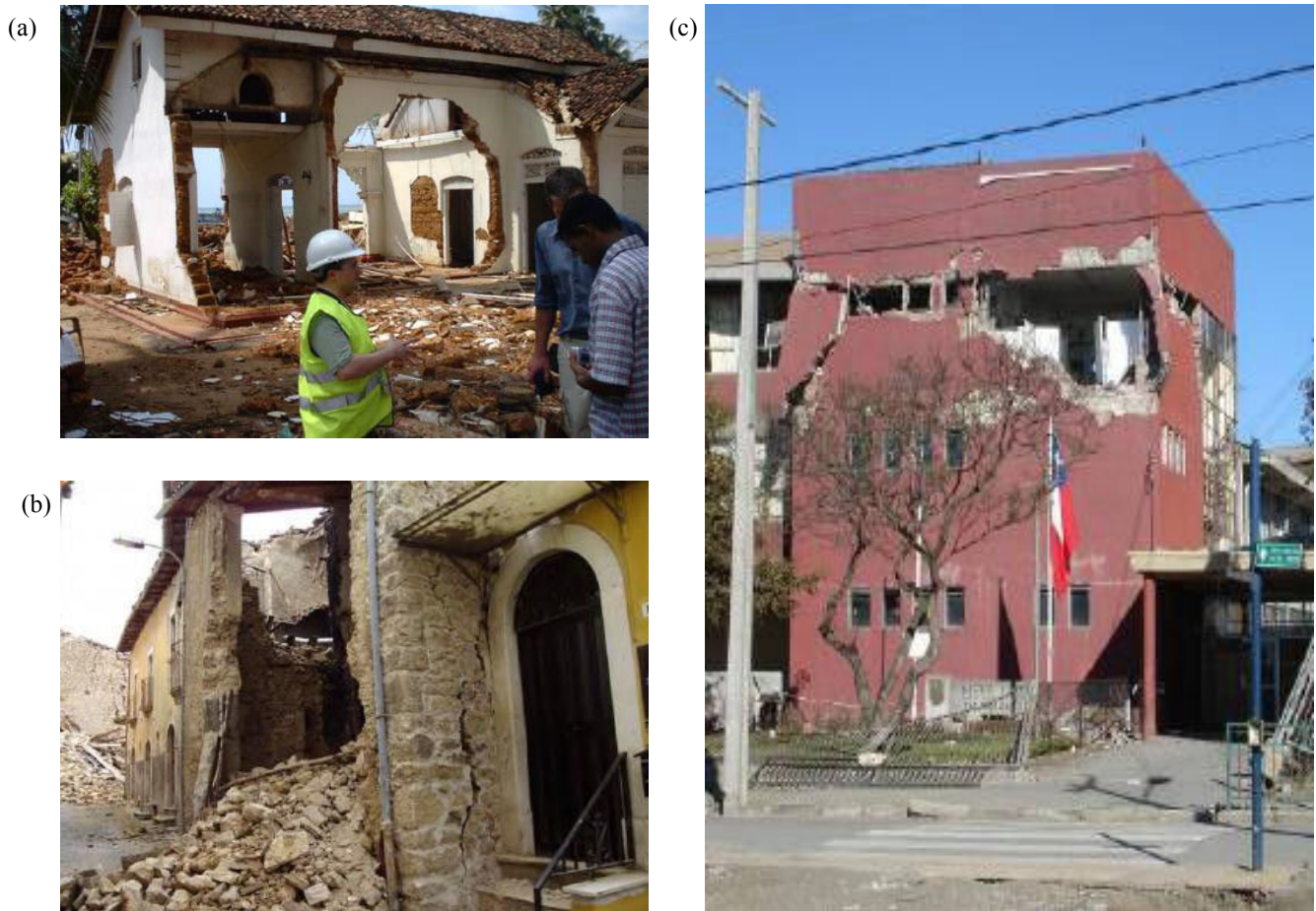
Fig. 10 Examples of damaged and collapsed building structures documented in reports by EEFIT (a) Tsunami damage to a residential building in Kalutara, Sri Lanka [32] (b) Earthquake damage to a traditional residential building in San Gregorio, Italy [41]. (c) Earthquake damage to a school building in Talcahuano, Chile [35]
