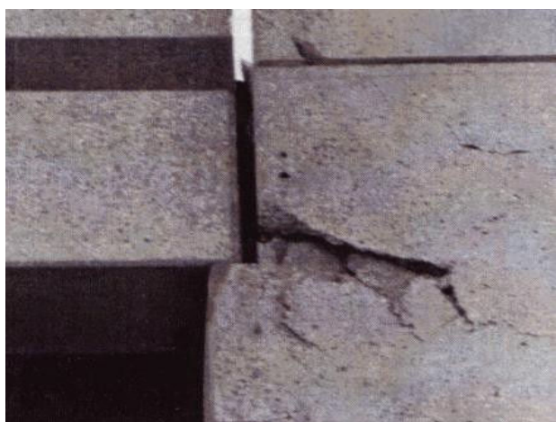
Fig. 8 Example of cracking of a precast concrete support of a parking structure documented in the ATC-20 series [29]
