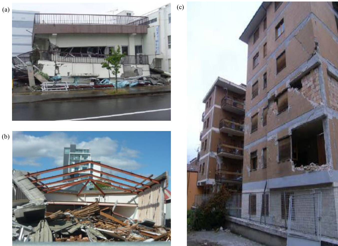
Fig. 11 Examples of damaged and collapsed building structures documented in reports by EEFIT and other publications (a) A collapsed office building in Oroshi, Japan [36]. (b) A partially-collapsed warehouse in Christchurch, New Zealand [39]. (c) Earthquake damage to an apartment block in L'Aquila, Italy [41]
