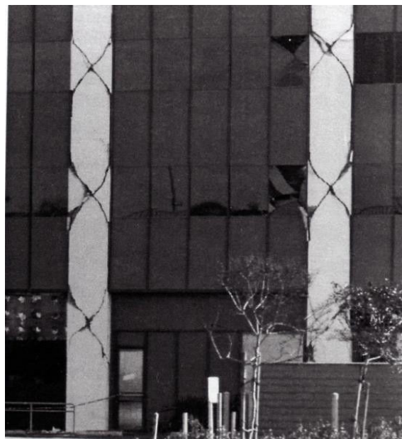
Fig. 9 Example of failed concrete piers (x-cracks) of a multi-storey building documented in the ATC-20 series [29]
