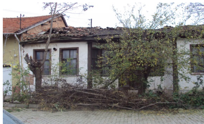
Fig. 2 A house about to collapse Karaagac – Edirne
