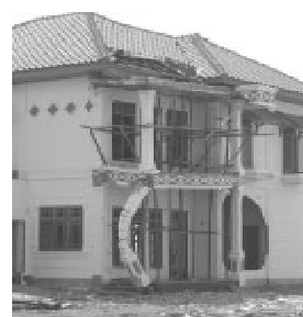
Fig. 1 Damage on a column due to tsunami waterborne object [3]
