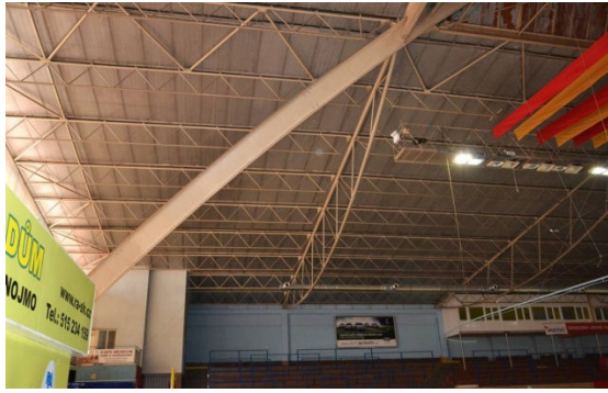
Fig. 7 Part of tested structure: truss main roof girders, truss purlins, bracings, arch main girders
