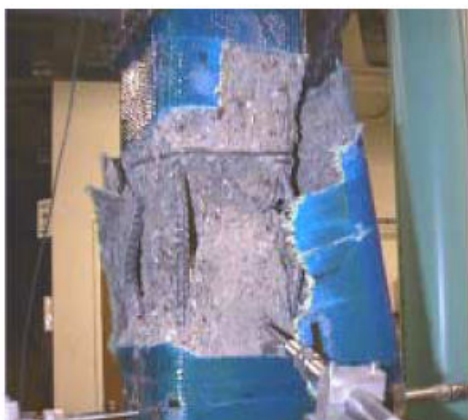
(b) Real cracks distribution [12]
