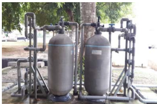
Fig. 2 The Water-Filter Tank installed outside the Canteen of Nilai University (inside the campus)
