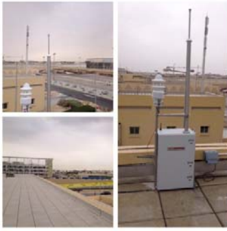
Fig. 2 The second monitoring station installed at a background location at the north from the first station
