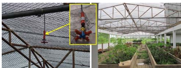
Fig. 5 The Fogger Installed Inside the Greenhouse
