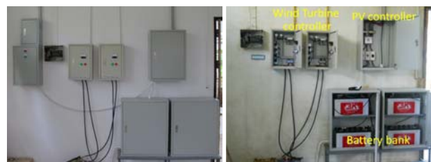
Fig. 4 The PV-Wind Charger and Controller and Battery Bank Installation
