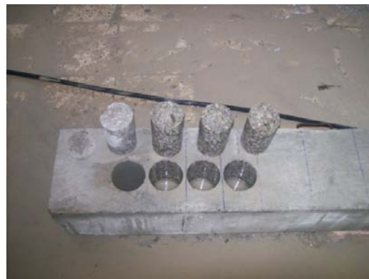
Fig. 3 Core samples taken from a reinforced concrete beam
